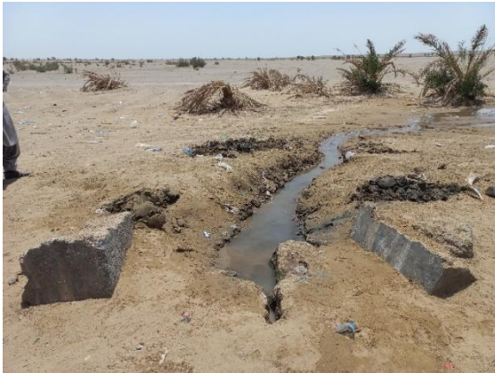
Destroyed Borehole NK9-MB
