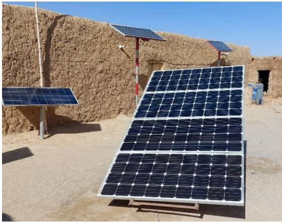
Solar Panels at Humai Settlement
