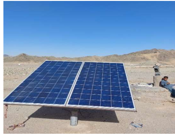
Solar Panels at Darband Chah Settlement
