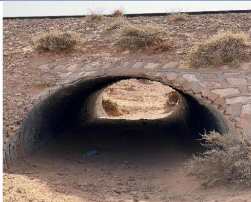
Figure 7.13 - Ø2400 mm Armco pipes under the railway line installed on the north-western boundaries of the project site
