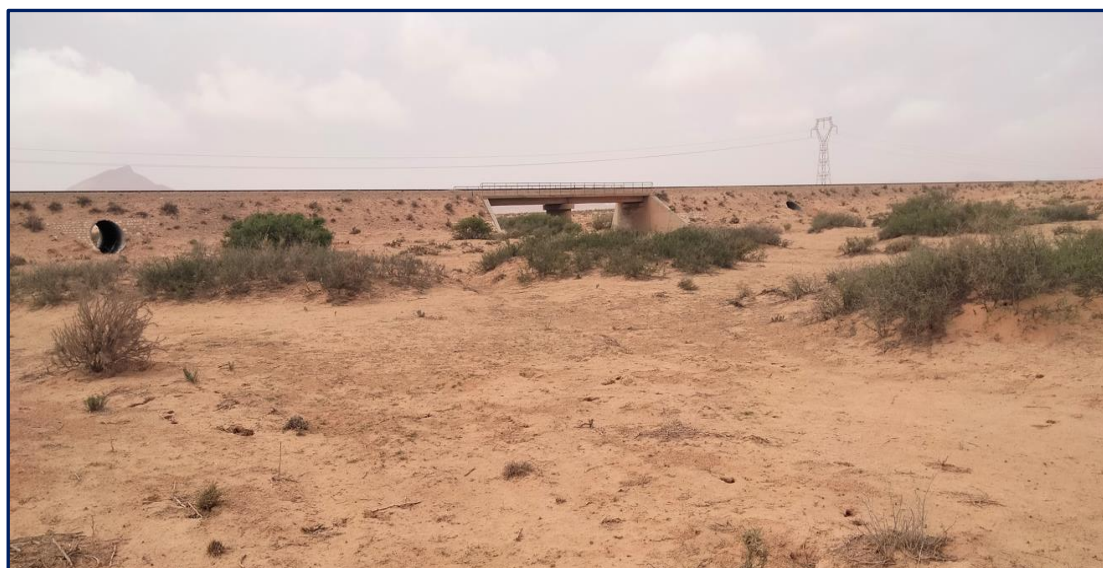
Figure 7.9 - Armco pipe Ø2400 mm and bridge with two spans of 11.6 m each
