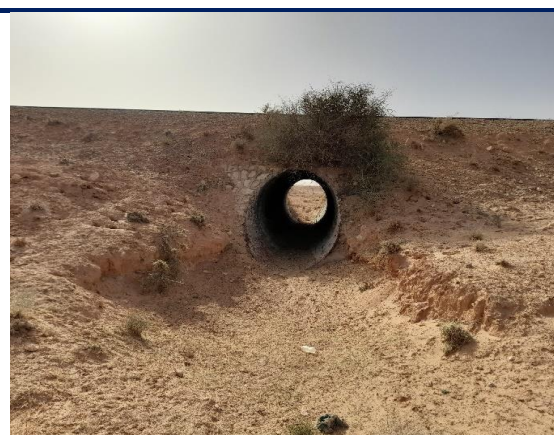
Figure 7.12 - Armco pipe Ø2400 mm on either side of the bridge
