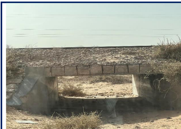
Figure 7.11 - Culverts (2.0 x 1.1) under the railway line upstream of the central part of the project site
