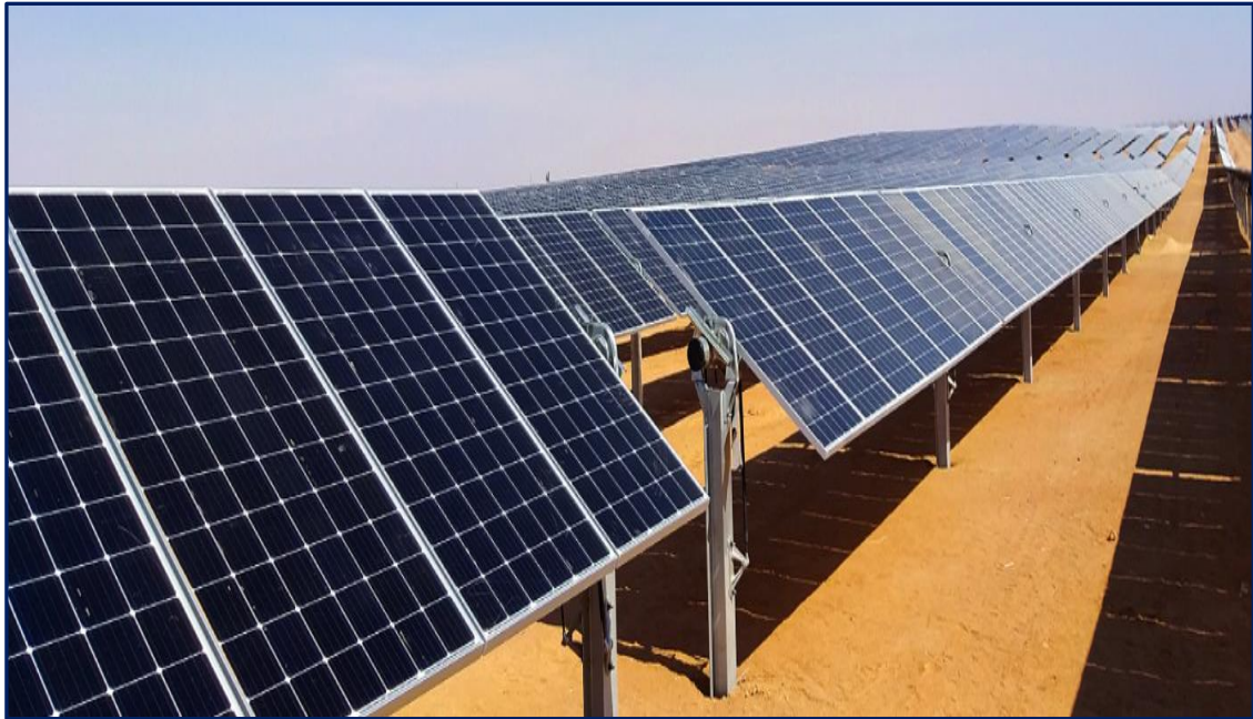
Figure 2.8 - Example of rows of PV panels
