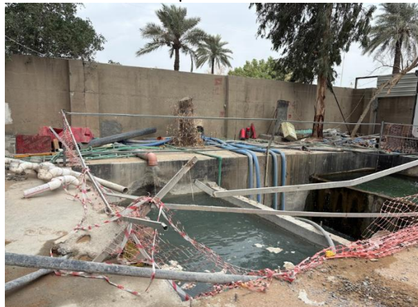
Groundwater abstracted is filtered and drained to Baghdad Municipality drainage
