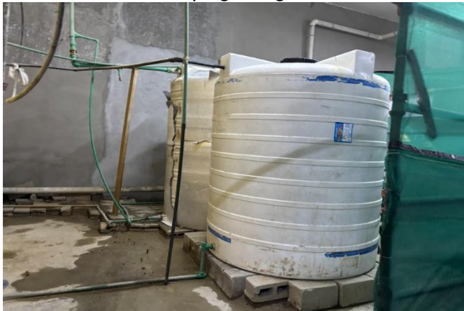
Raw Water Storage Tank
