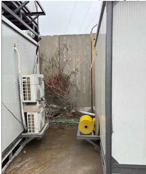
Sewer pipelines passing adjacent to porta cabins and being drained at Municipality drainage
