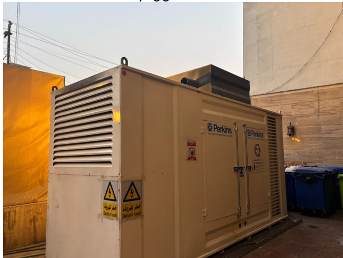
DG set at Labour camp
