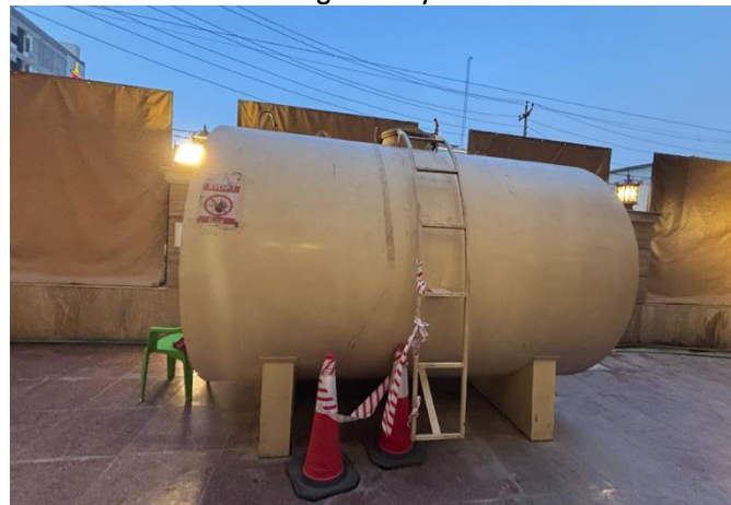
Diesel Fuel Tank at Labour camp
