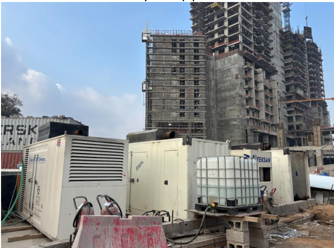
Diesel Generators at Ground Floor
