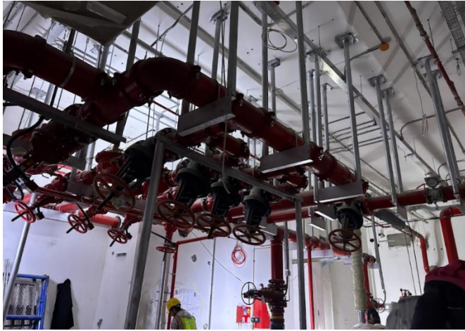
Fire hydrant pipeline
