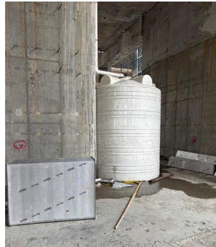
Construction wastewater collection tank on each floor
