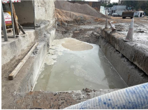
Concrete mixing wastewater slurry stored in a pit near Batching plant area
