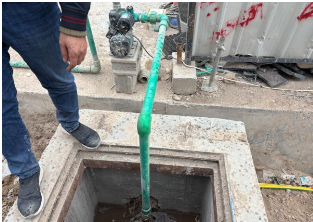
Water meter installed in pipeline
