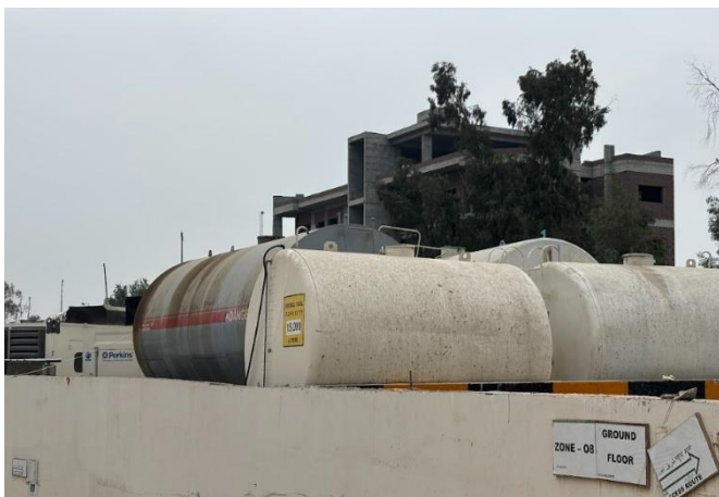
Diesel Fuel Tankers at Ground Floor
