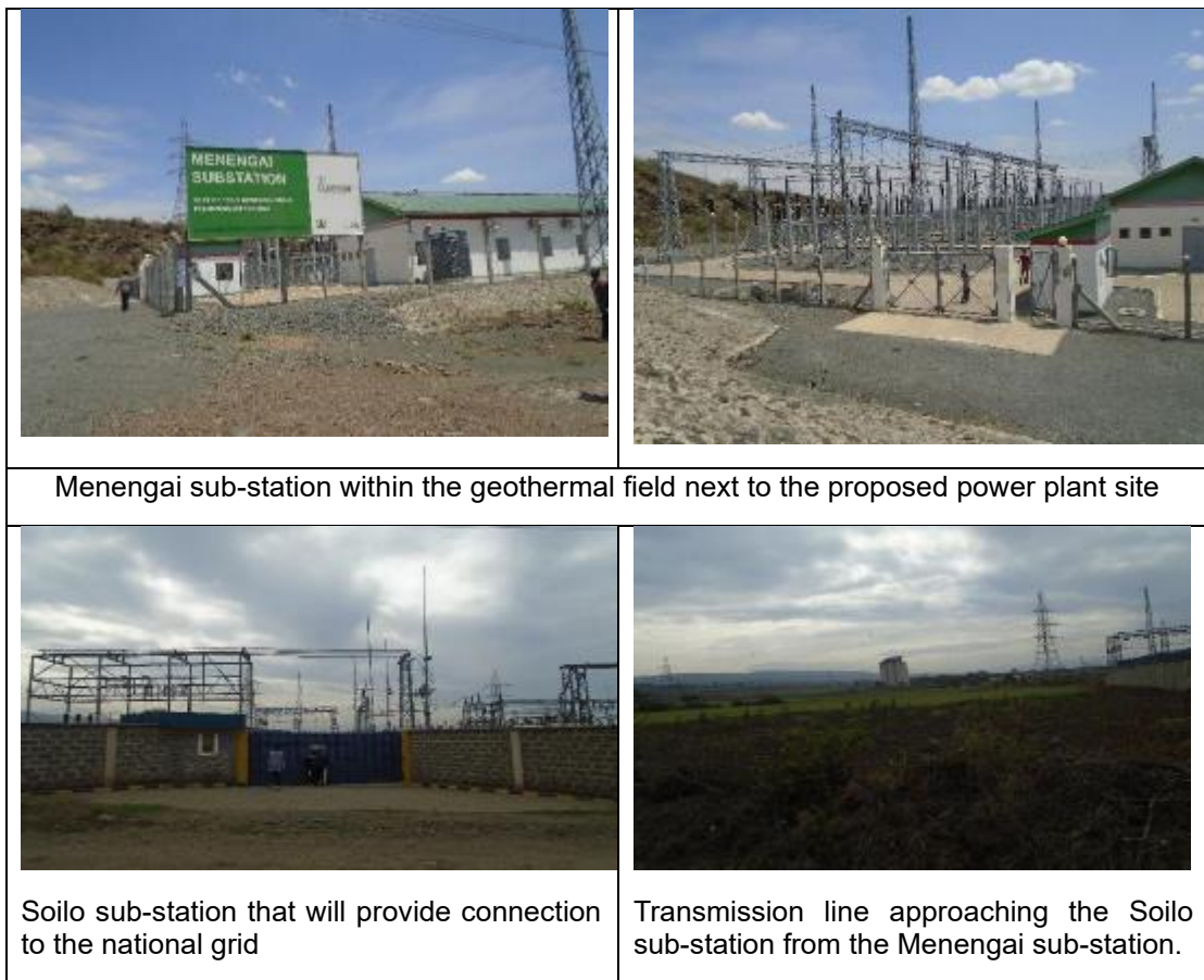
Photo 4-1: KETRACO Substations and transmission line within the project area of influence
