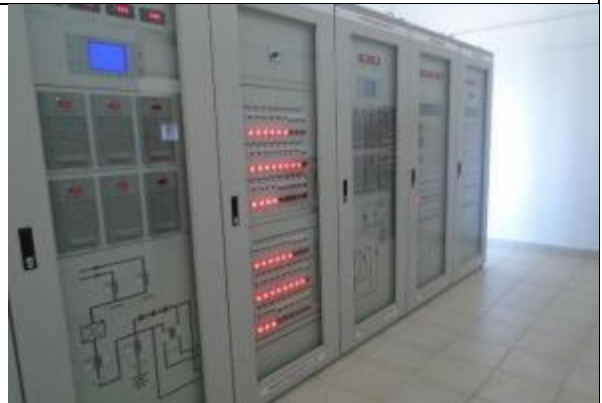
Control room at the Menengai Sub-station
