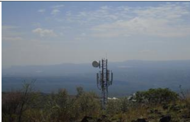
A telecommunication mast near the view point/Mlima punda
