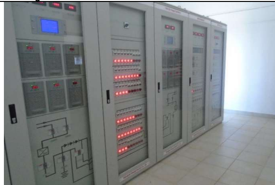
Control room at the Menengai Sub-station
