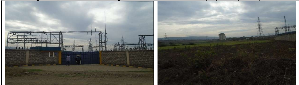
Soilo sub-station that will provide connection to the national grid
