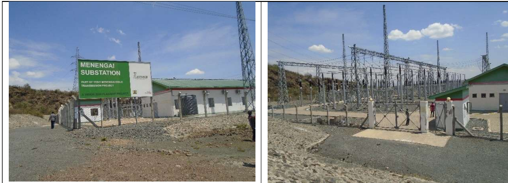
Menengai sub-station within the geothermal field next to the proposed power plant site
