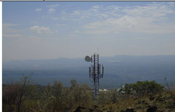
A telecommunication mast near the view point/Miima punda
