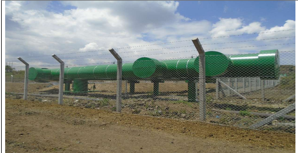
OTTL, Quantum and Sosian steam interphase point with the GDC installed steam gathering system
