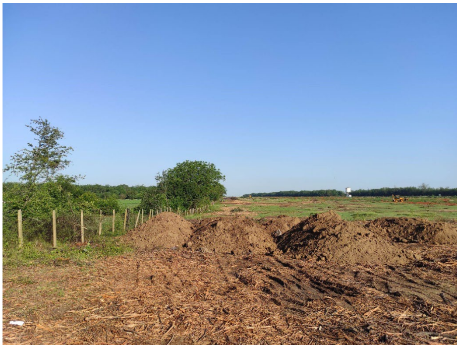
Figure 21: Final removal of tree and shrub vegetation along northern and southern airport boundaries, buffer strips and self-established vegetation around the airport runway – May 2023.
