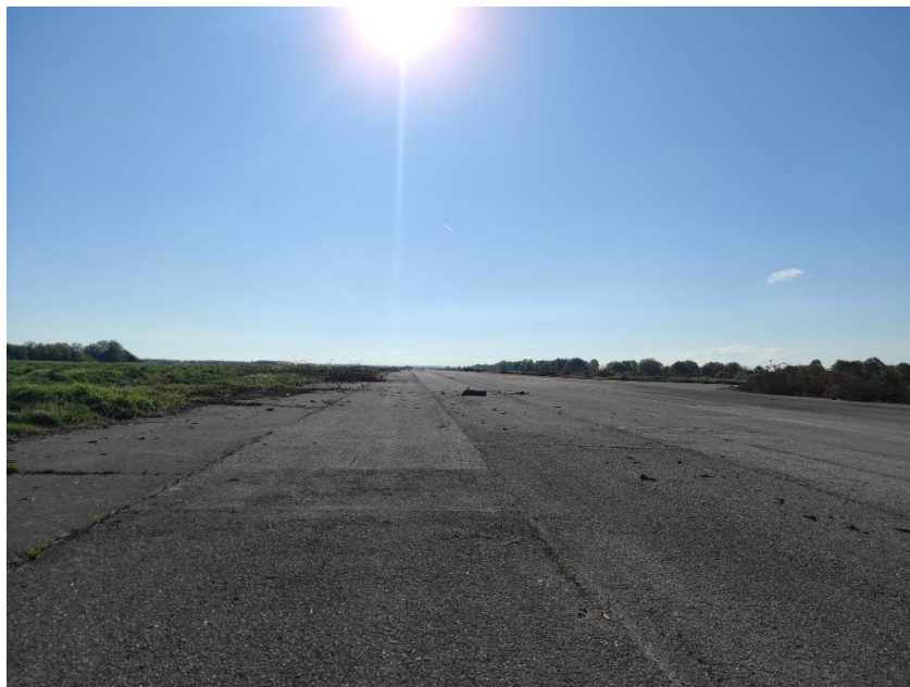
Figure 3: Missing tree and shrub vegetation around the track – May 2023.
