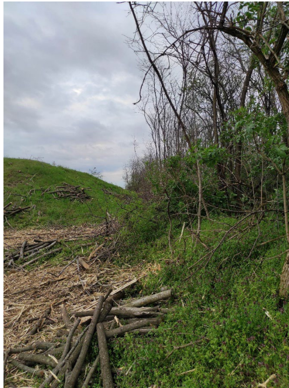
Figure 20: Beginning of felling of tree and shrub vegetation along the northern and southern borders of the airport – March-April 2023.
