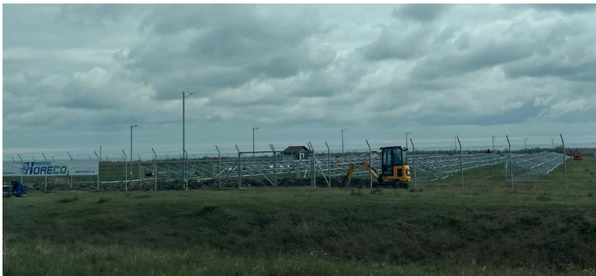
Figure 7-6 Photovoltaic power plant in Costesti
