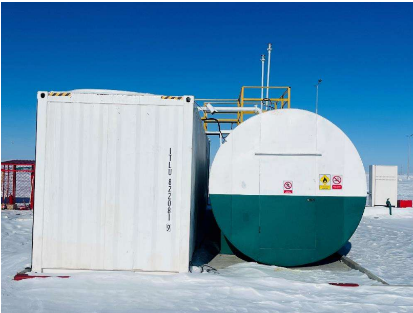
Figure 69. Relocated main fuel tank at Farming Complex, February 2024
