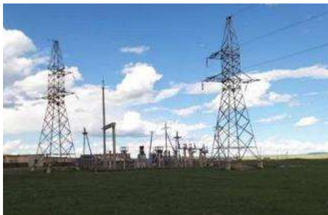
Figure 79. Ulziit village substation. Ecotrend
