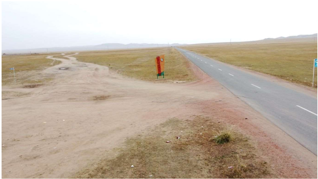
Figure 3. Unsealed edge of carriageway
