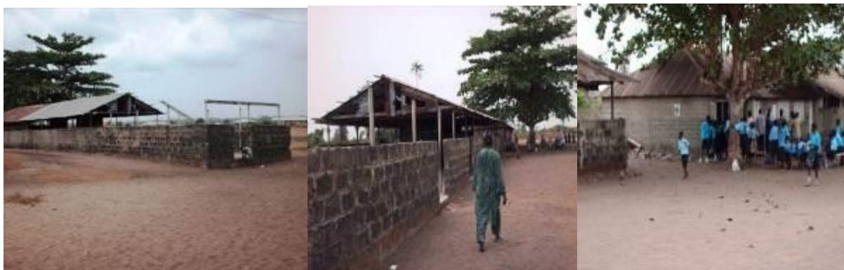
Plate 4.24: Back and side-views of the post primary school infrastructures for the Community High School (CHS), Idotun, showing the level of deterioration
