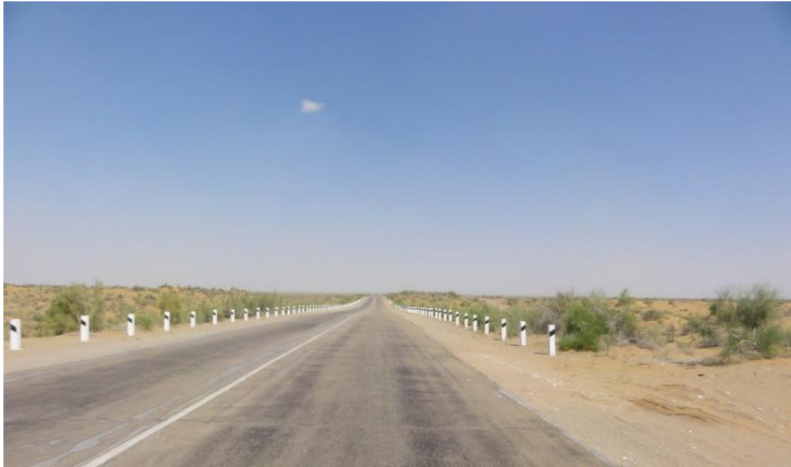
Figure 8-1: Road Condition A739 North of Zarafshan 104
