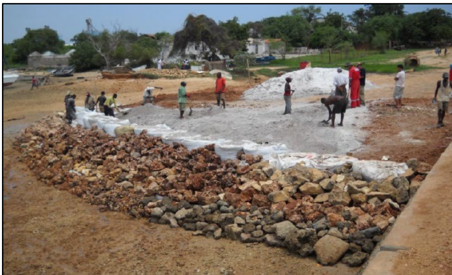
Figure 24: Construction of a temporary jetty using gravel, sandbags and rocks to armour
