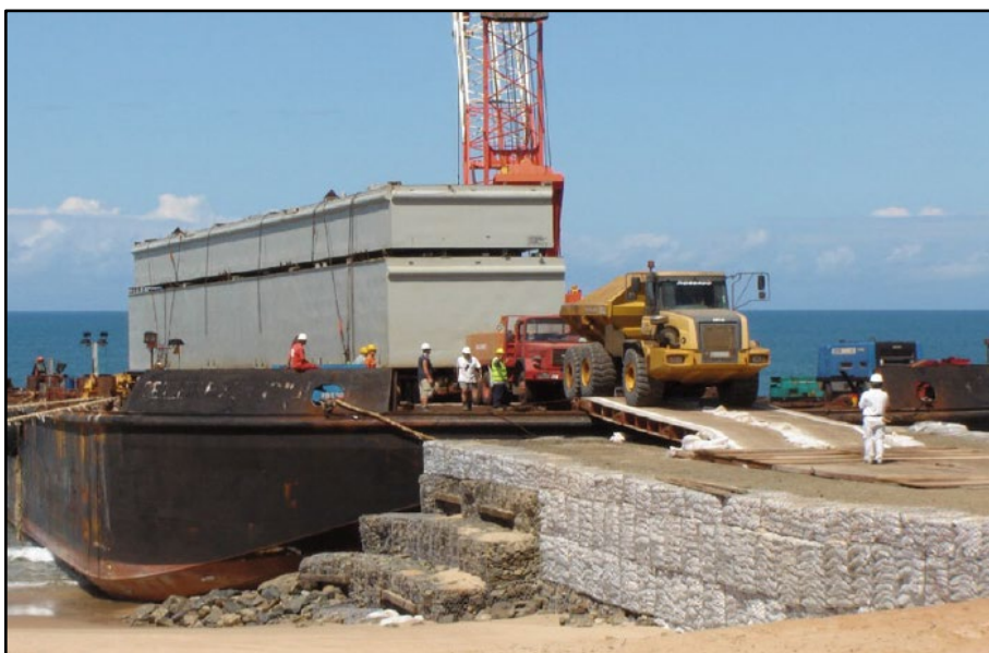
Figure 25: Example of a temporary jetty (gabions) during offloading from barge, with barge lying on the sand bed.
