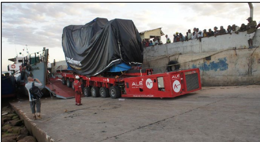
Figure 30: Equipment mounted on self-propelled modular transporter being driven off the barge at temporary jetty
