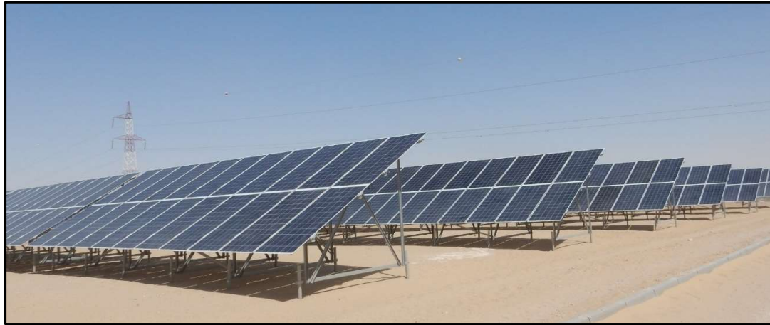
Figure 2.4 - Typical Power Arrays Composed of PV Panels
