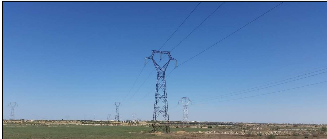
Figure 2.5 - Typical HV Lines
