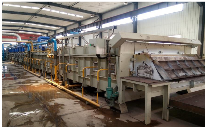
Plate 4: Typical On-line Annealing Furnace
