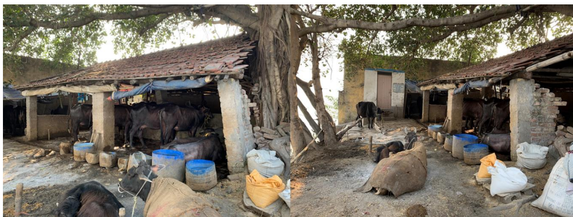
Figure 4.1 Structural Impact on Cattle Shed in Bally
