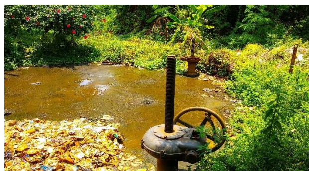
Grid Chamber at Arupara PS
