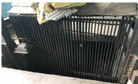
Grid Chamber at Ichapur MPS
