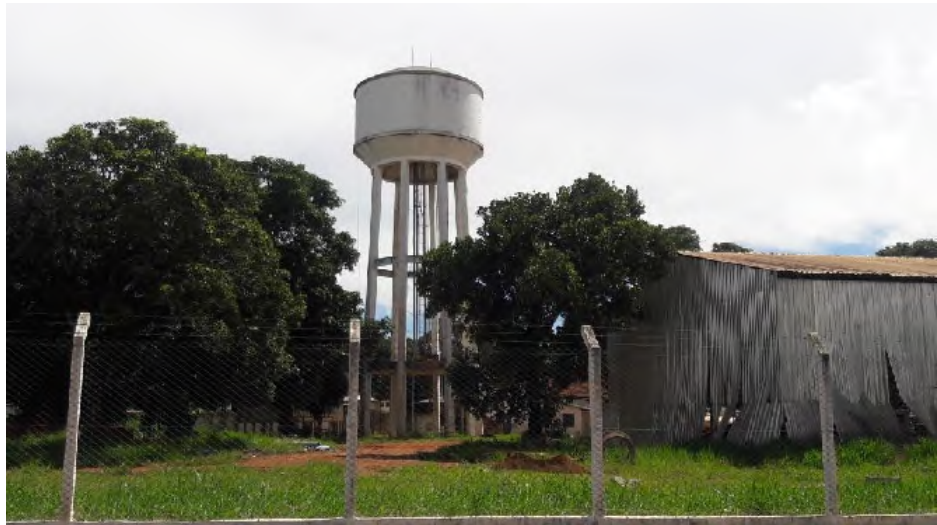
Figure 37 – SAE water tank in Araguari. Source: Pöyry Tecnologia (2018).
