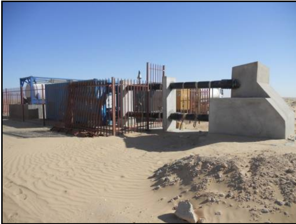
Photograph 3-9: Borefield Pumping Station (located along access road)
