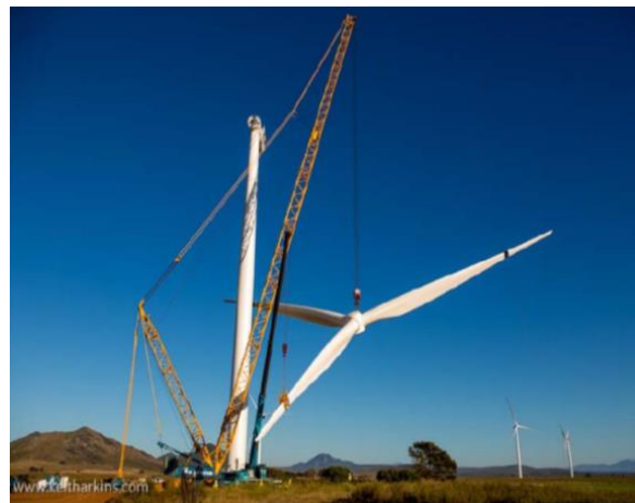
Rotor Lift: crane supporting blade tip until necessary ground clearance is achieved.
