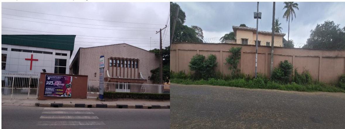
Plate 3.8: Images showing affected fences at Ilsamaja and Ilupeju areas Source: Sustainabiliti Limited, September 2022
