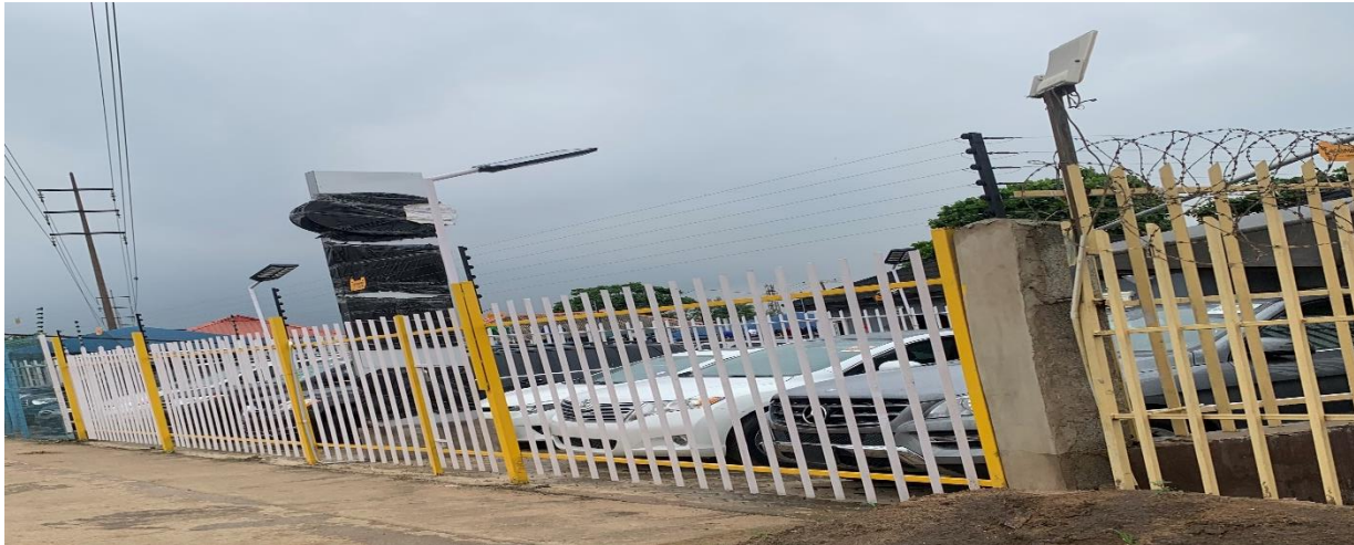
Figure 3- 4: Shows the affected metal fence wall at a proposed layby. Source: LAMATA, July 2023.
