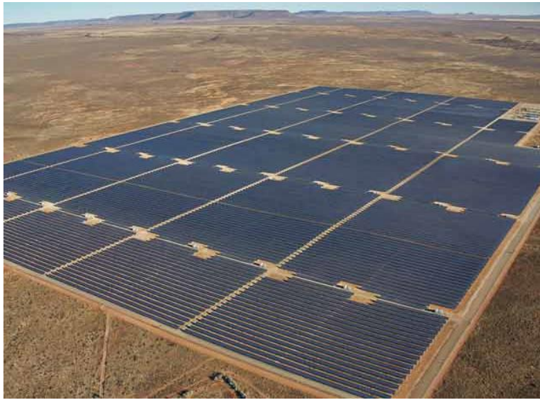
Figure 11. Typical PV Power Arrays Composed of PV Panels
