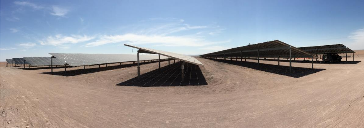
Figure 63. Atacama Pilot PV plant
