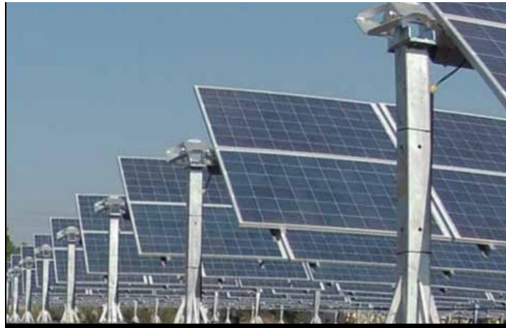
Figure 10. Horizontal-axis tracker system
