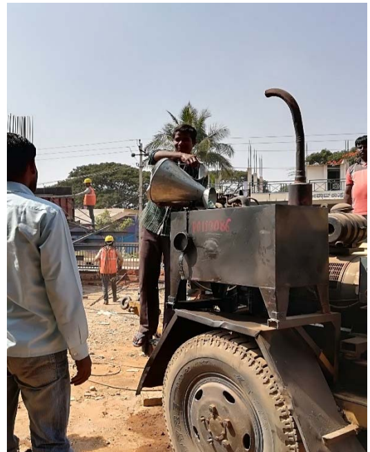
Photo 24: Workers without relevant PPE at Kushtagi flyover construction site
