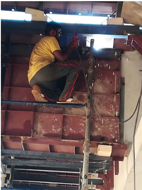
Photo 23: Workers working without adequate PPE at Kushtagi flyover construction site
