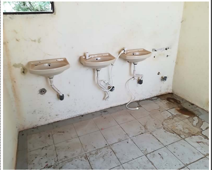
Photo 18: Wash basin in wayside amenities
