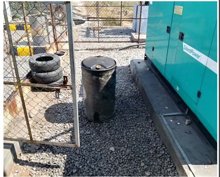
Photo 6: Oil spill and stain at DG set Operation
