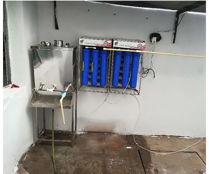
Photo 8: RO Plant at Toll Plaza
