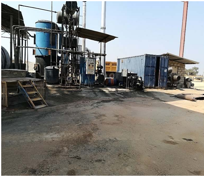
Photo 9: Stains of oil spills
