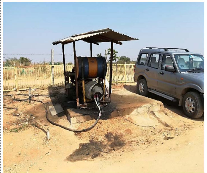
Photo 10: Oil spill at DG and DG set without Acoustic enclosures
