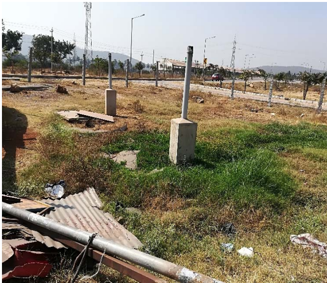
Photo 27: Damaged septic Tank at Toll Plaza
