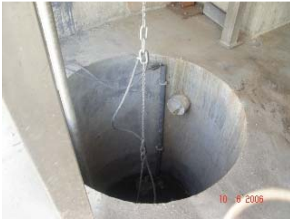
Photograph 4-7: Wastewater Influent Pit
