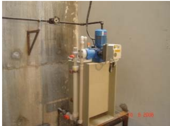
Photograph 4-10: pH control (Acid Dosing)
