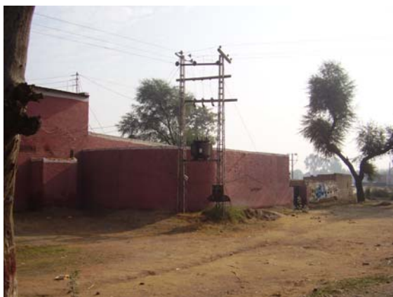
Transformer and power transmission line at existing factory
