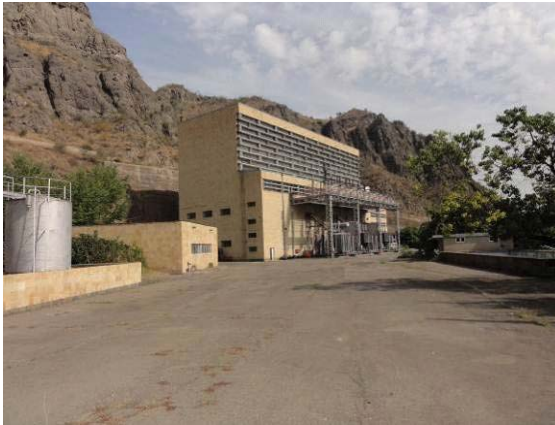
Photo 63: Rocks falling down regularly to HPP site after heavy rain
