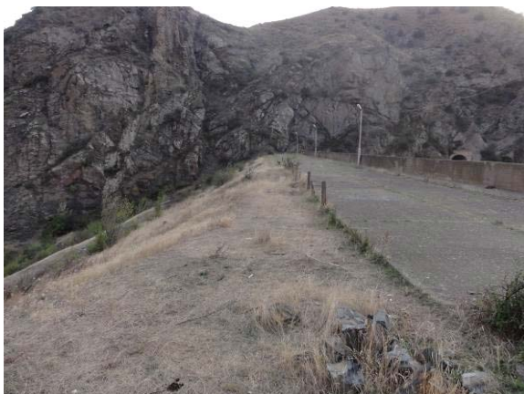
Photo 30: No wall or balustrade on downstream side of dam
