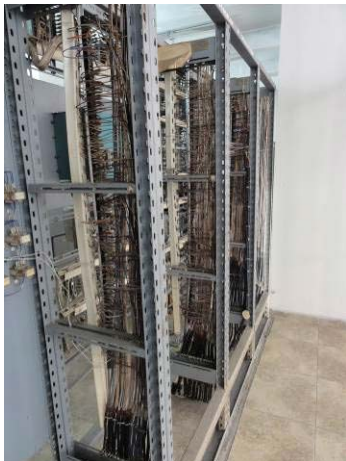
Photo 49: Open backside of electric devices
