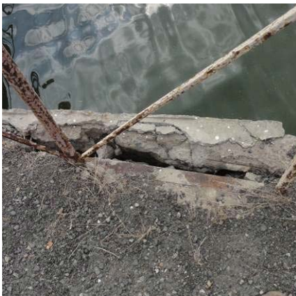
Photo 38: Fixing of handrails is breaking
