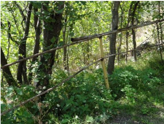
Photo 15: Handrails near gate broken
