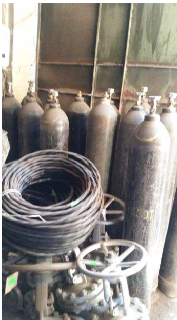
Photo 74: Gas cylinders not safely stored
