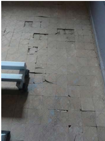
Photo 47: Floor in battery room broken and not acid proof
