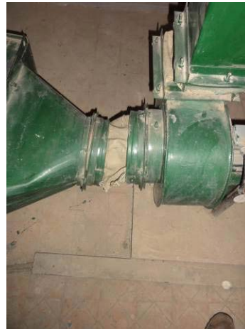
Photo 48: Ventilation system of battery room not working
