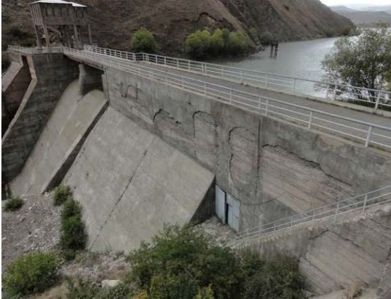
Photo 11: Concrete wall of dam damaged; tunnel entrance
