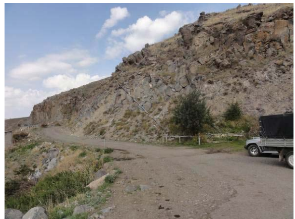
Photo 2: Rocks above access road to be secured by nets
