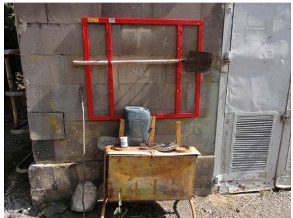
Photo 20: Missing firefighting equipment
