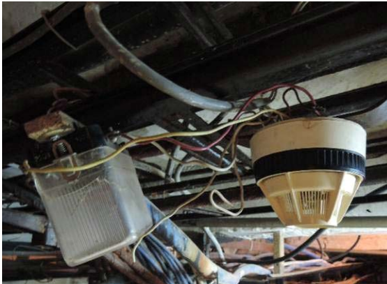
Photo 59: Fire alarm system in bad condition
