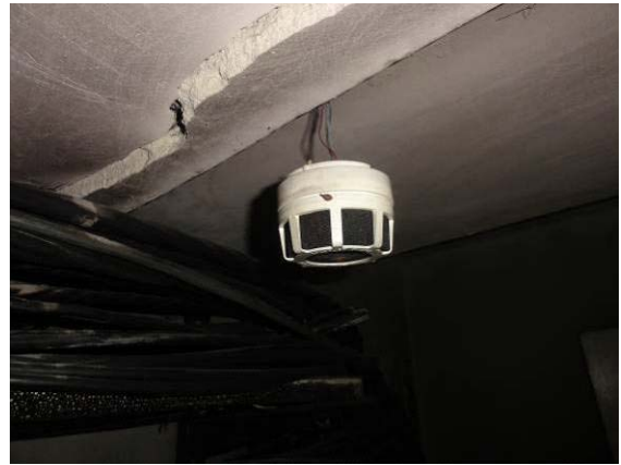
Photo 46: Fire alarm system not working
