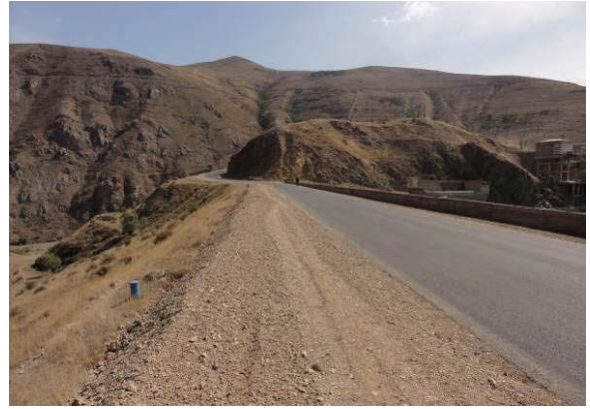
Photo 25: No wall or balustrade on downstream side of dam
