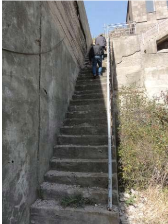
Photo 17: Stairs and handrail to tunnel damaged
