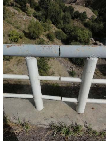
Photo 12: Handrails at dam are broken
