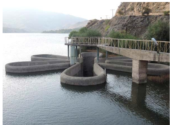
Photo 31: Unsafe handrails at dangerous overflow installation
