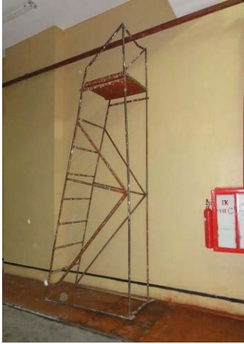
Photo 68: Unsafe device for working at height
