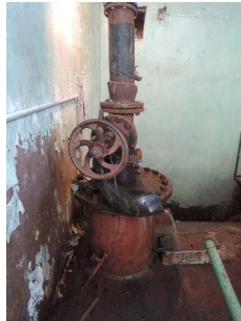
Photo 79: Technical equipment needs refurbishment
