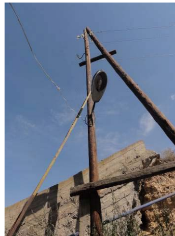
Photo 27: Outside illumination not working
