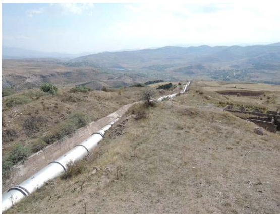
Photo 76: Over ground pipe between Spandaryan Reservoir and Spandaryan HPP
