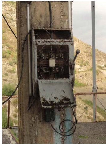
Photo 41: Unsafe electrical installations
