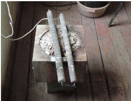
Photo 19: Unsafe heating device
