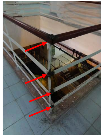
Photo 50: Unsafe welded handrails
