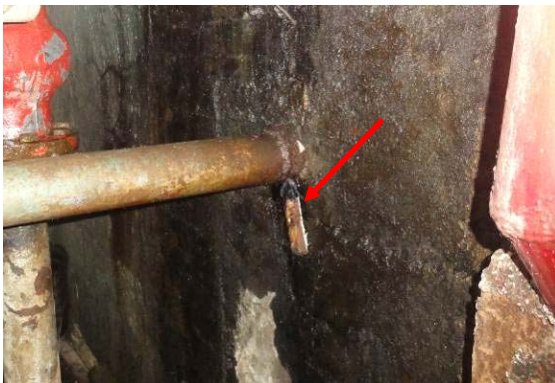
Photo 65: Oil leakages fixed with wooden wedges
