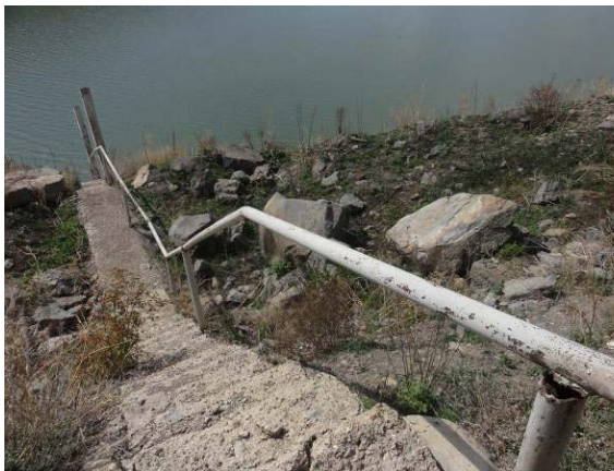
Photo 3: Stairs and handrails damaged by falling rocks
