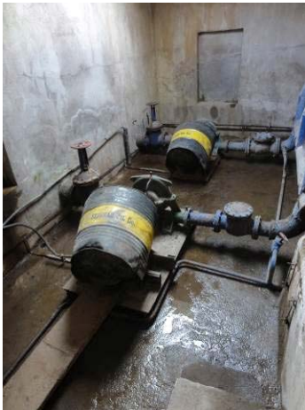
Photo 53: Installations of firefighting system are very old and need refurbishment
