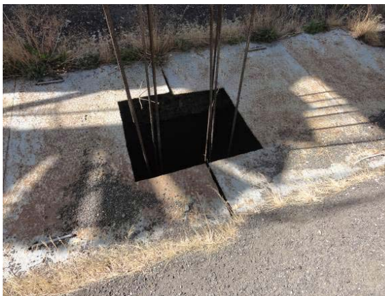
Photo 21: Weak and unsafe metal sheets
