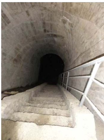
Photo 23: No illumination in tunnel (gallery)
