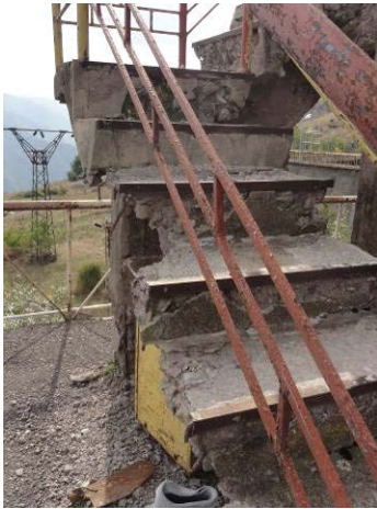
Photo 40: Unsafe and broken stairs and handrails
