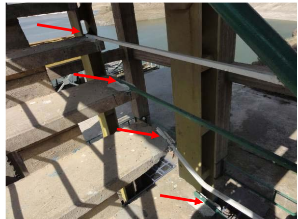
Photo 29: Self-repaired unsafe stairs and handrails at intake control building
