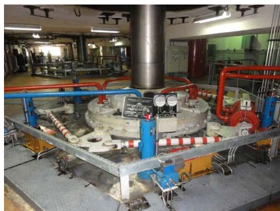
Photo 66: Lack of guarding at rotating machinery
