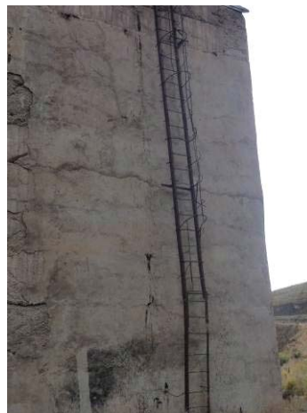
Photo 10: Dangerous ladder outside outlet control building
