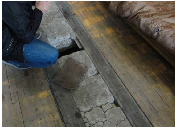
Photo 60: Holes in floor in restroom
