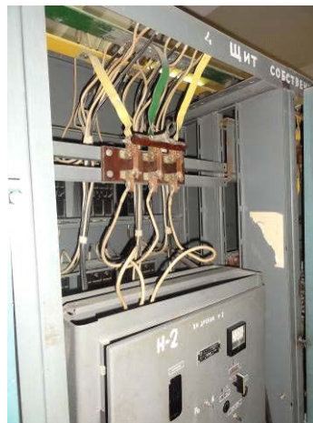
Photo 62: Unsecure electrical devices
