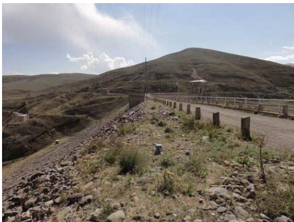
Photo 1: No handrail or wall at downstream side of dam
