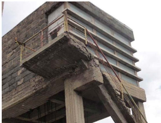
Photo 39: Unsafe and broken stairs and handrails
