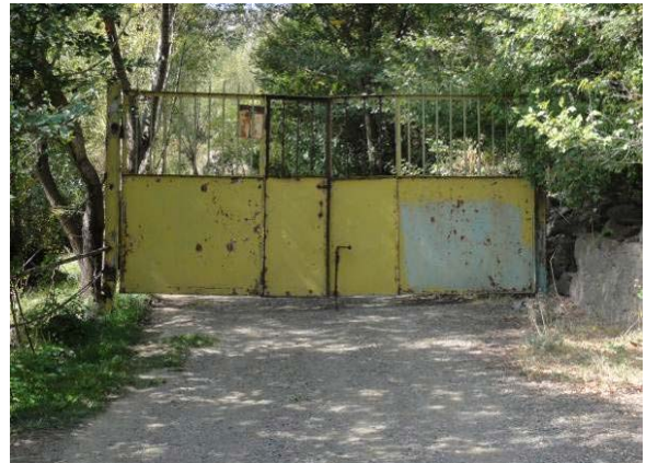
Photo 16: Entrance gate in bad condition
