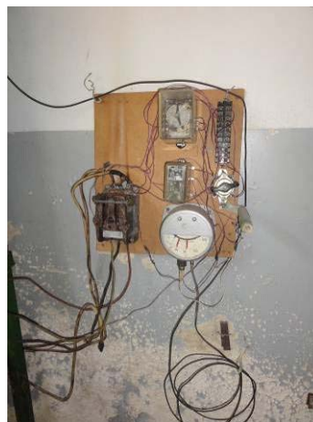
Photo 67: Unsafe electric installations
