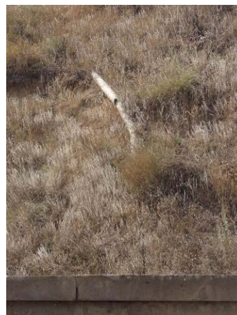
Photo 43: 6 kV cable mantled with asbestos
