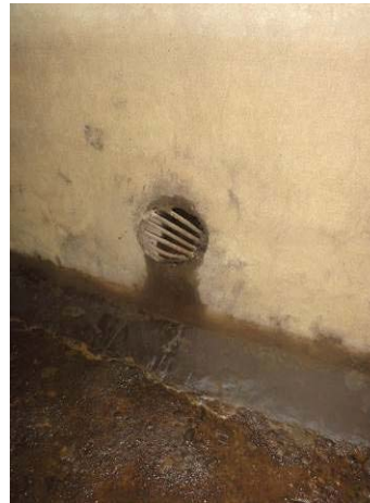
Photo 54: Water intake for firefighting system about 50 cm above ground of outlet channel
