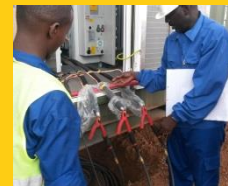
Medium voltage final tests
