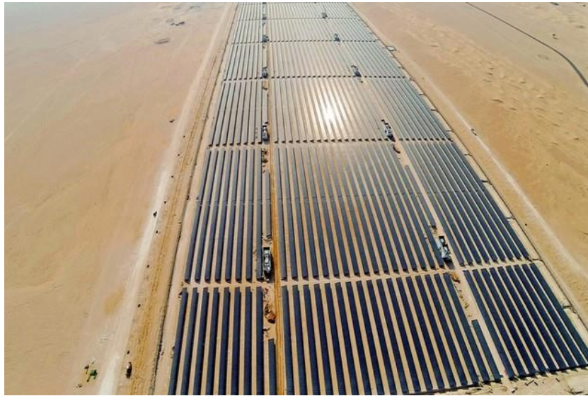
Figure 10. Typical PV Power Arrays Composed of PV Panels
