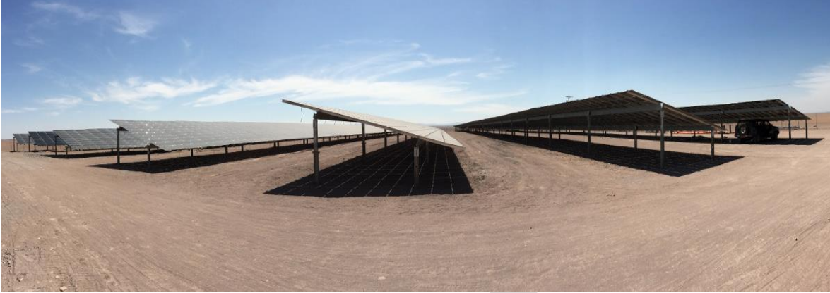
Figure 58. Atacama Pilot PV plant
