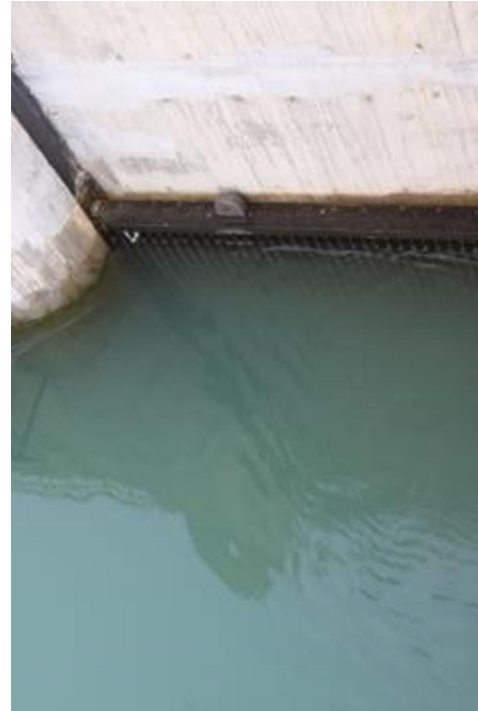
Photo 4: Otluca HEPP - Intake Protection Grill
