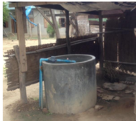
Water supply (Sa Khar village)
