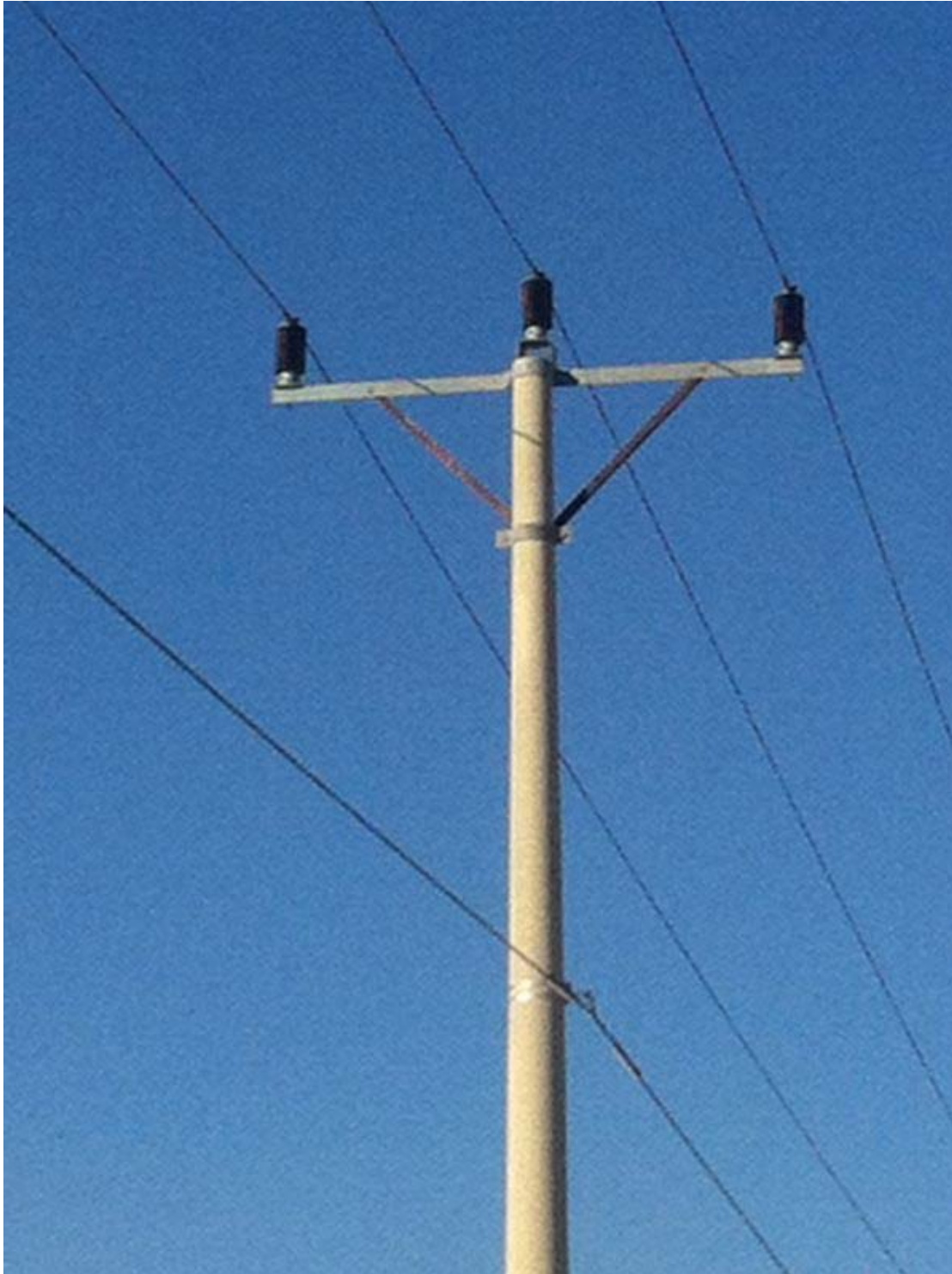
Figure 3.2.2: A transmission Line of 33 Kv
