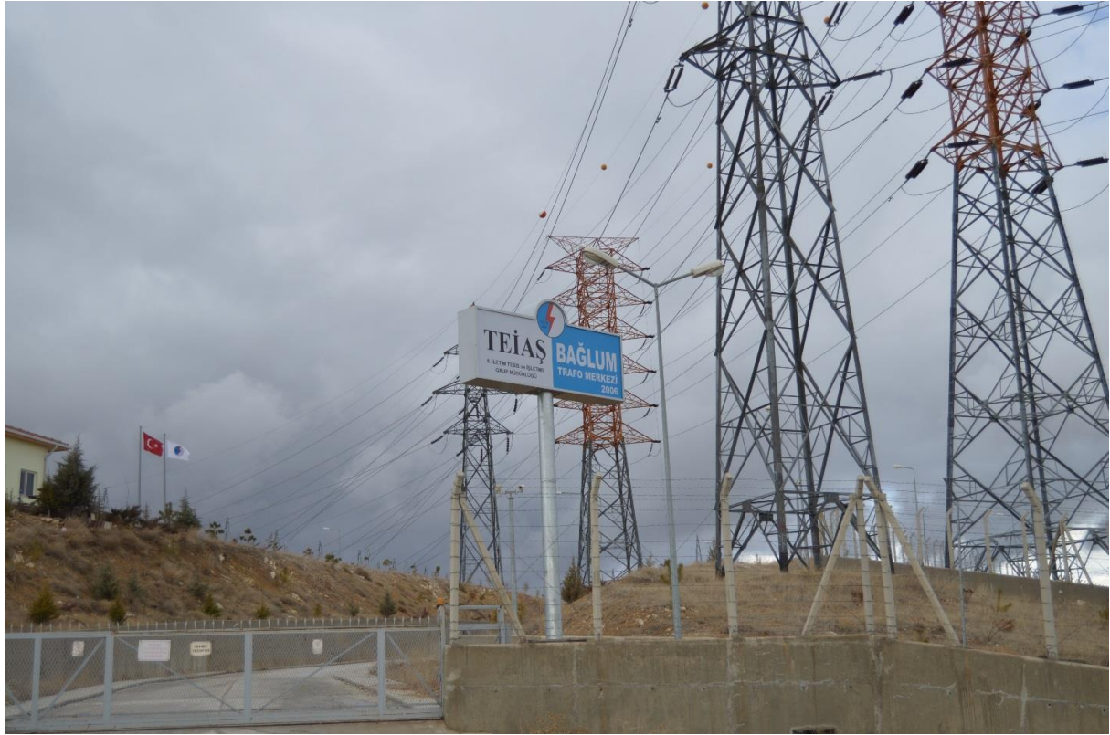
Figure 5. Photograph of the Project Area (Bağlum Substation)
