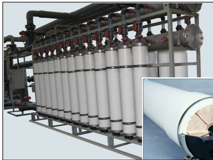
Figure 66. An Example of Ultrafiltration System
