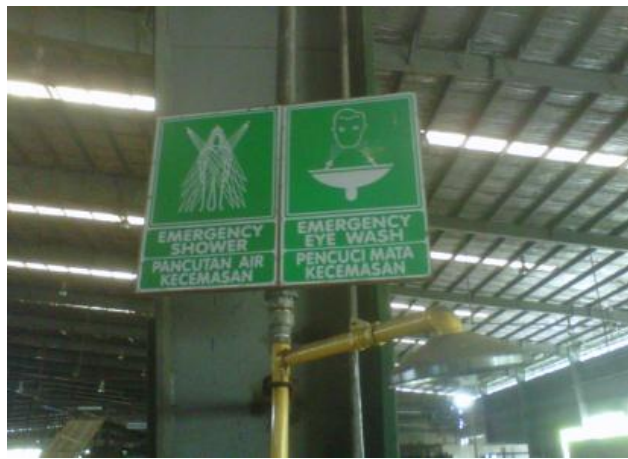
Photo 19: Emergency shower/eye wash system installed
