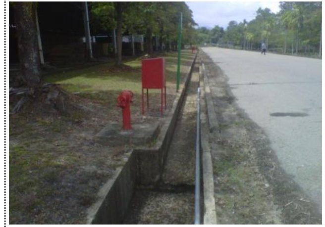
Photo 21: Hydrant system installed at ITC facility
