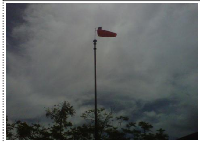
Photo 24: Windssock for wind direction and speed (important for detection of chemical leak)
