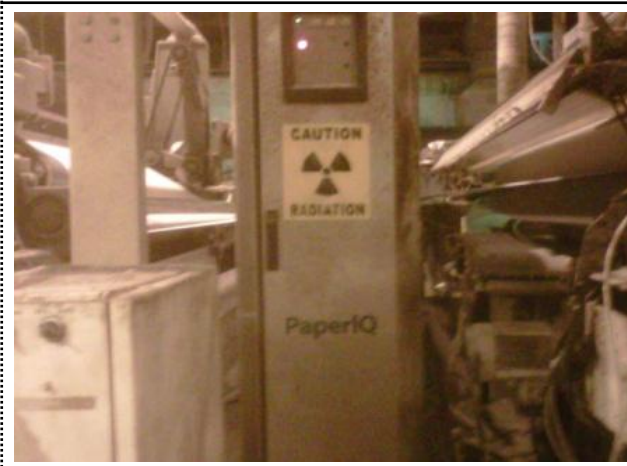
Photo 23: Signage at radiation zones. Necessary PPE designated for work in this area
