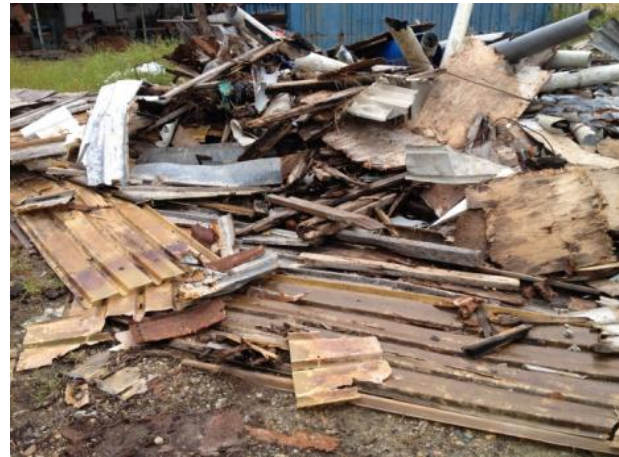
Photo 17: Improper disposal of friable asbestos
