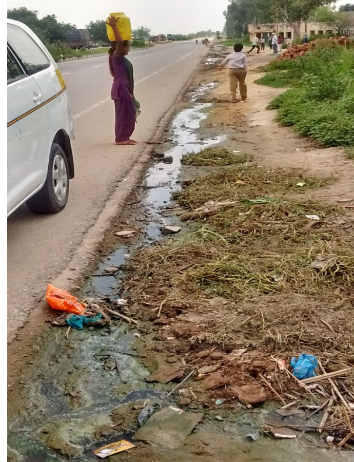
Photo 24: View of the poor maintenance of carriageway.
