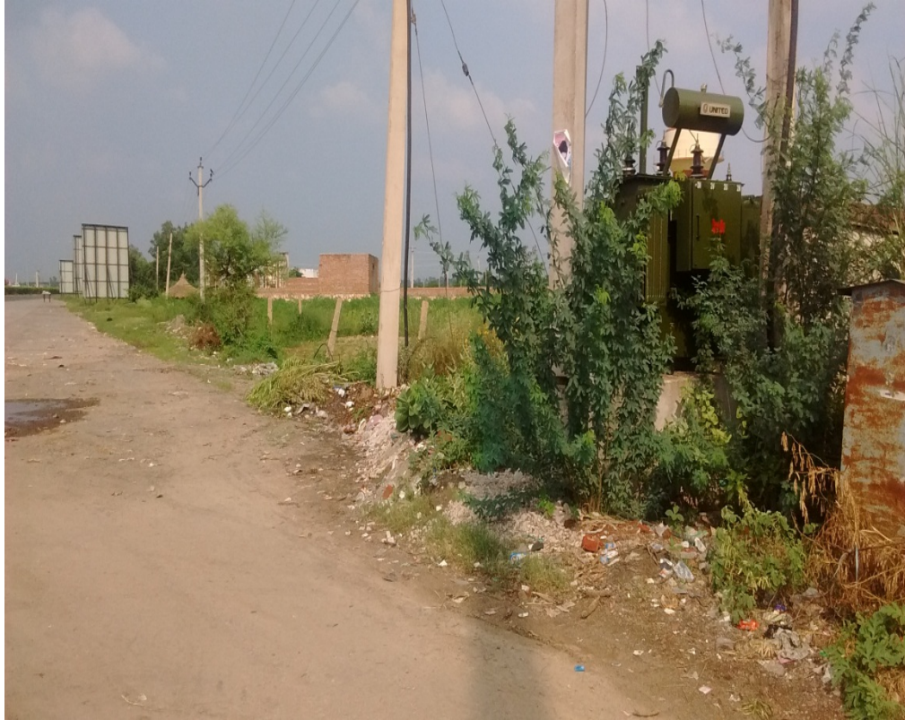
Photo 3: View of the poor ROW maintenance with no solid waste management
