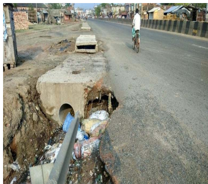
Photo 22: Solid waste within the ROW of project road
