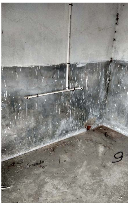
Photo 27: Incomplete water connection inside toilet at truck lay bye
