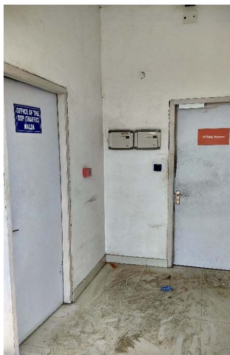
Photo 28: HTMS room at toll plaza
