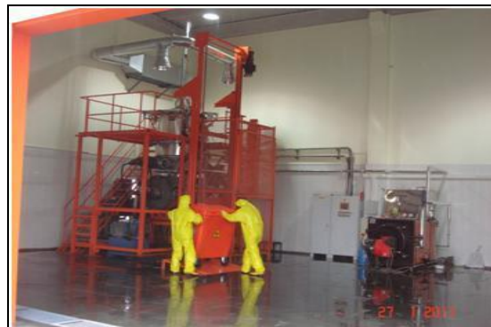
Photo 6. Medical waste sterilization unit
