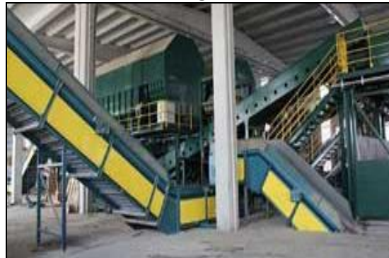
Photo 2. Waste sorting unit
