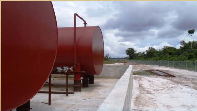
Fuel Tanks with Safe Containment
