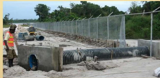
Fencing with Drainage
