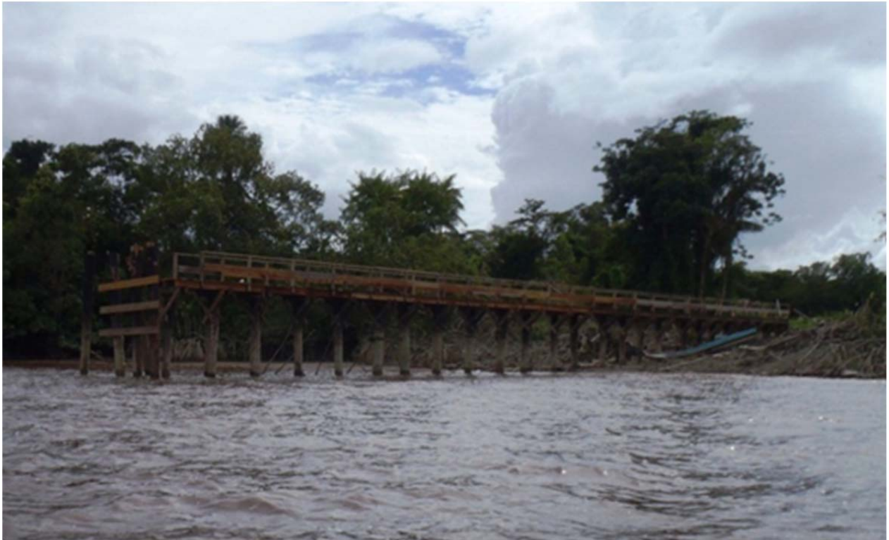
Figure 2.2-1: Fuelling Trestle, Buckhall Logistics Support Facility
