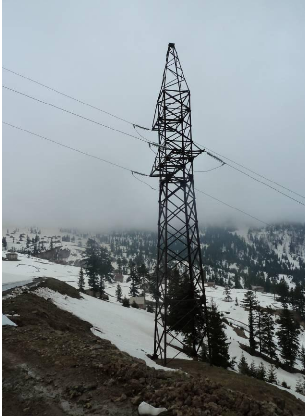
Figure 2.17: Existing 110 kV transmission line
