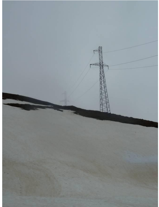
Figure 2.18: Existing 110 kV transmission line
