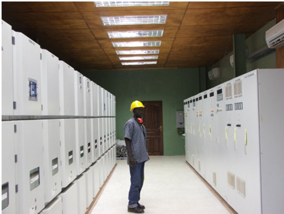
Figure 5-9: Image of typical LV switchgear (right) and MV switchgear (left)
