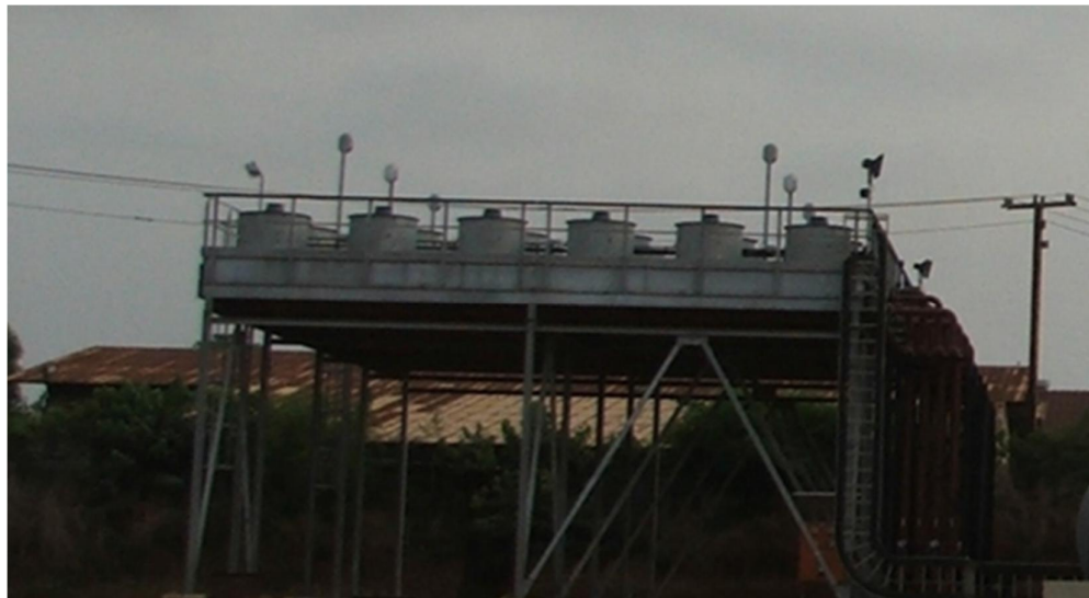
Figure 5-5: Typical image of radiators
