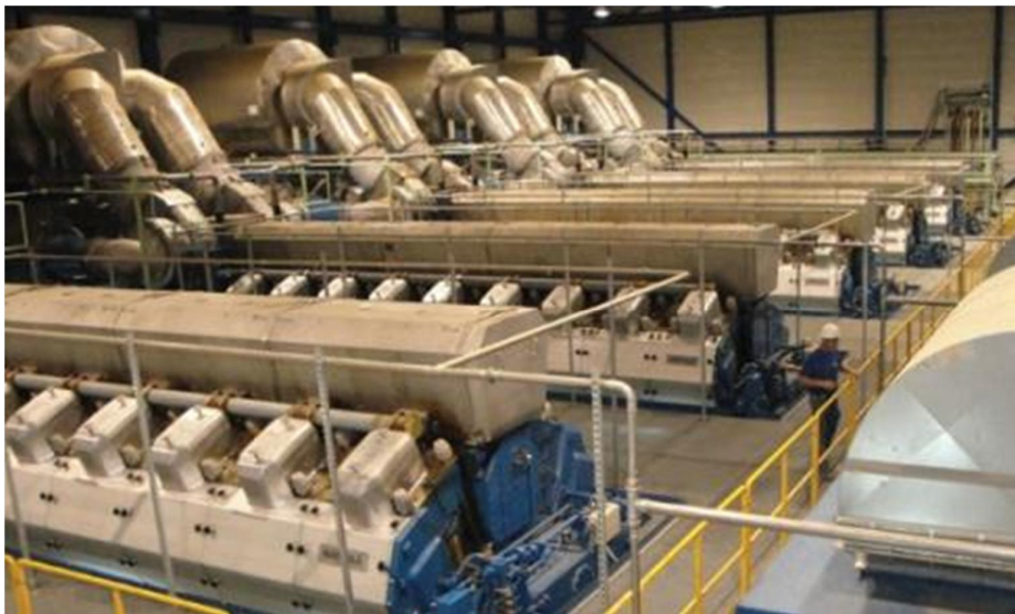
Figure 5-4: Typical image of power house with generator sets installed
