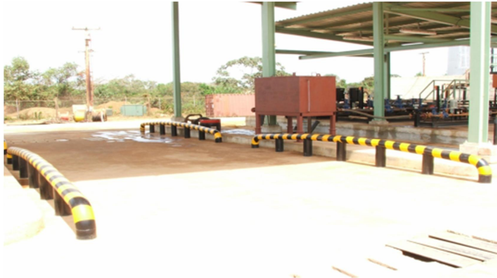
Figure 5-8: Image of a typical truck off-loading station
