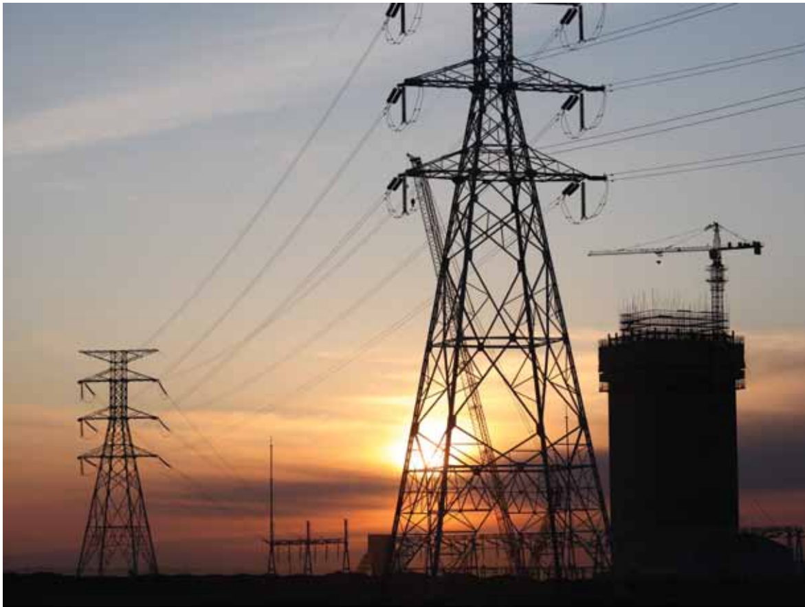
Initial power supply for the project will be imported from China via a new power line. Here the line passes in front of one of the shaft heads being constructed to access the underground deposits
