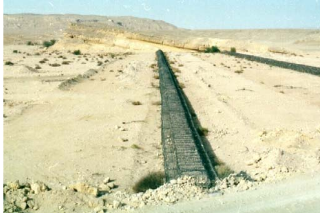
Figure 4-8: Two successive retardation dykes supporting one another, constructed at the narrow trunk of Wadi Ghweiba for flashflood protection
