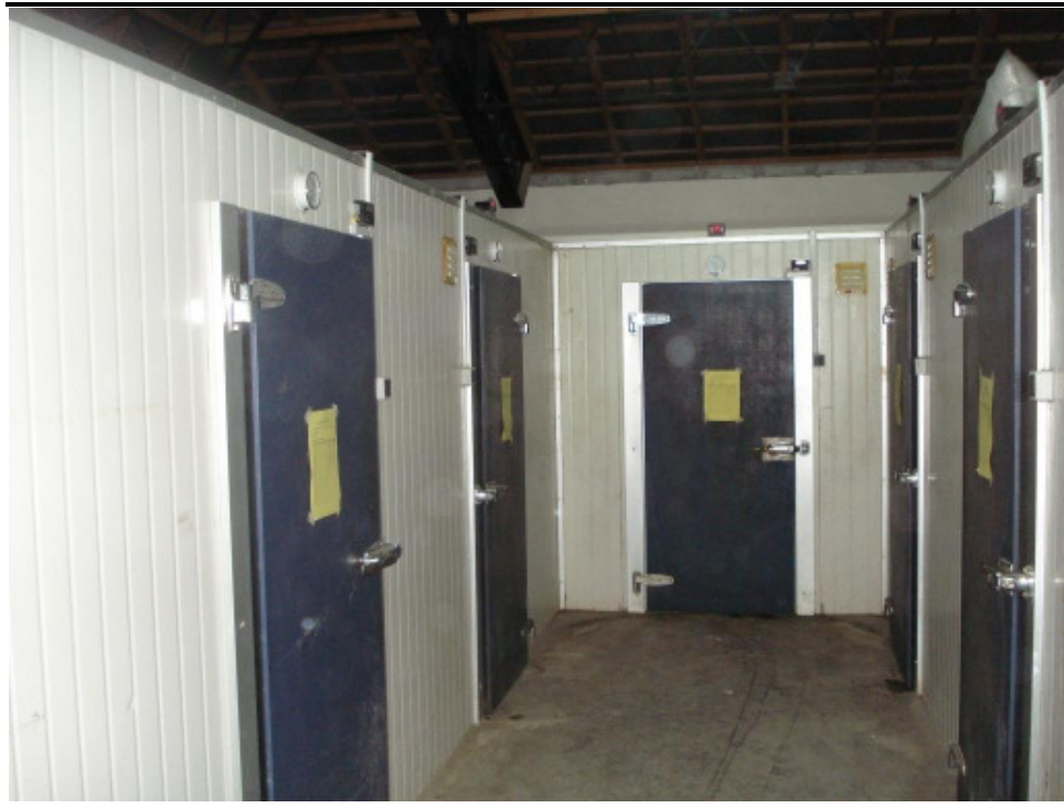
Photo 9 Blast Freezers and Cold Rooms
