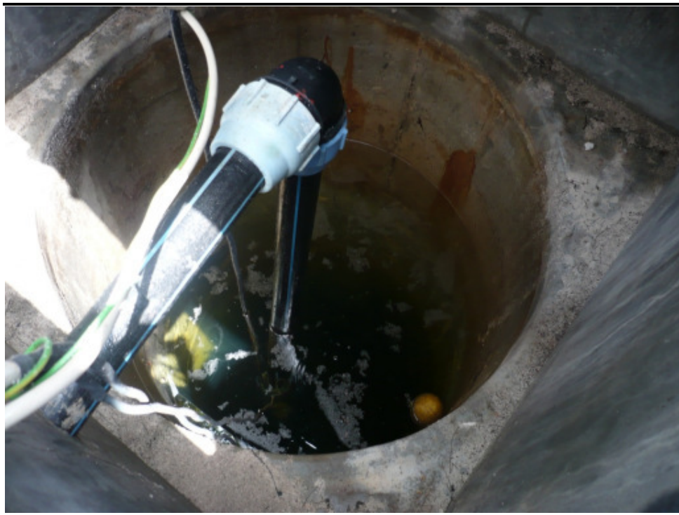
Photo 22 One of the boreholes used to draw water for the desalination plant
