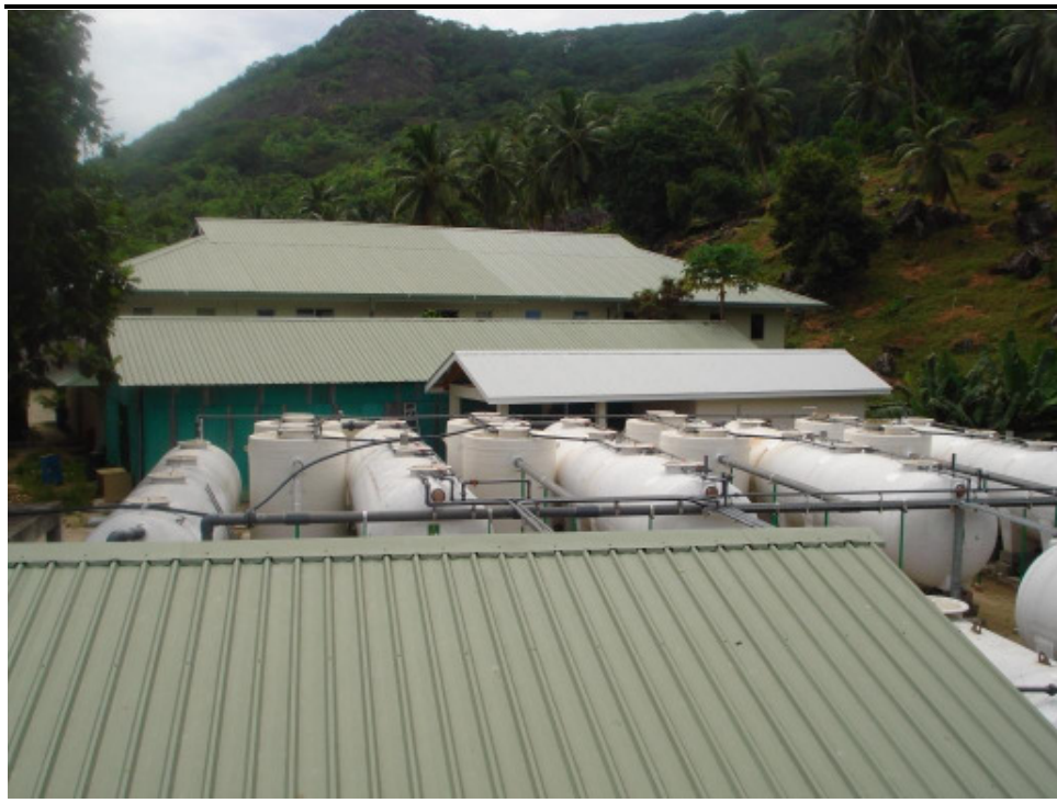
Photo 12 Sewage Treatment facility with maintenance roof in the background
