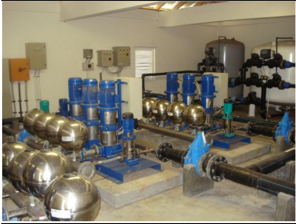
Photo 5 Potable Water Filtration and Pump room
