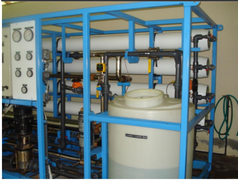
Photo 17 Reverse Osmosis Treatment Unit
