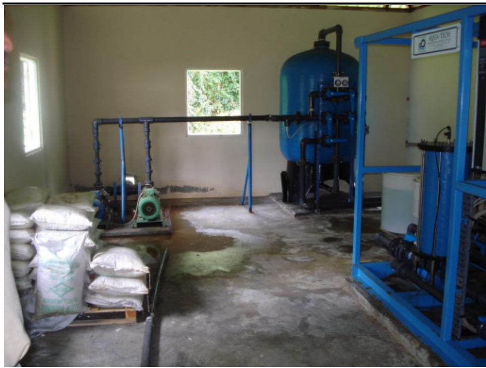
Photo 18 Reverse Osmosis Treatment Room
