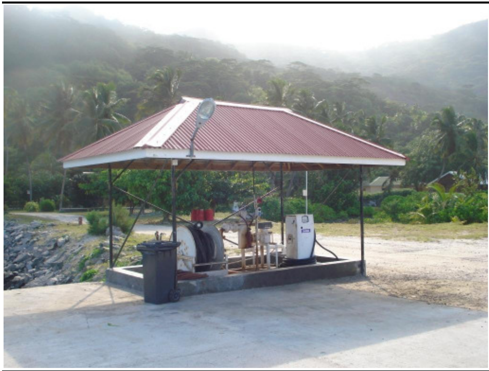
Photo 2 Fuel Pump Station
