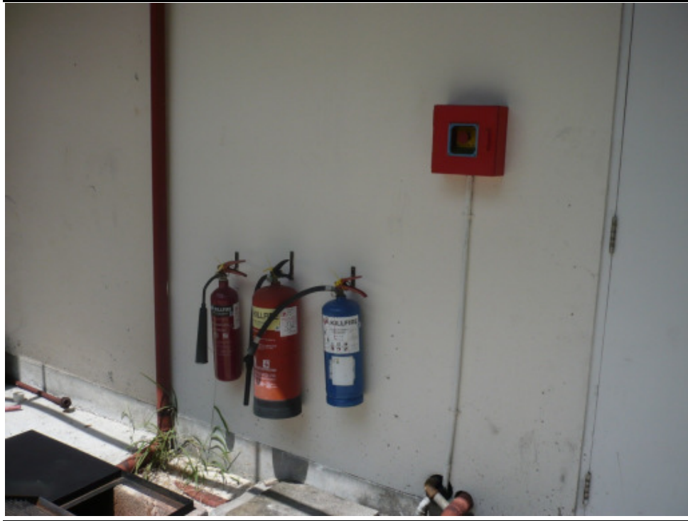
Photo 21 Fire-fighting equipment found at several locations on the Resort
