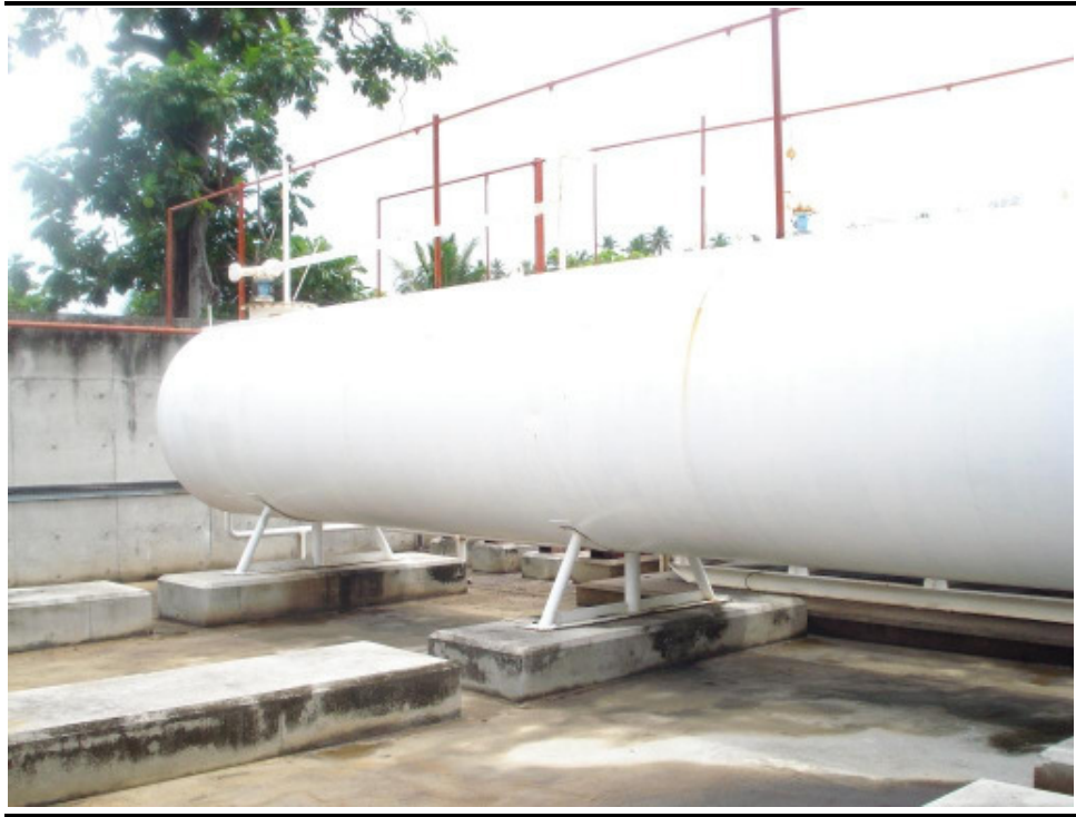
Photo 19 Bulk Diesel Storage Area showing - 40,000l Above Ground tank
