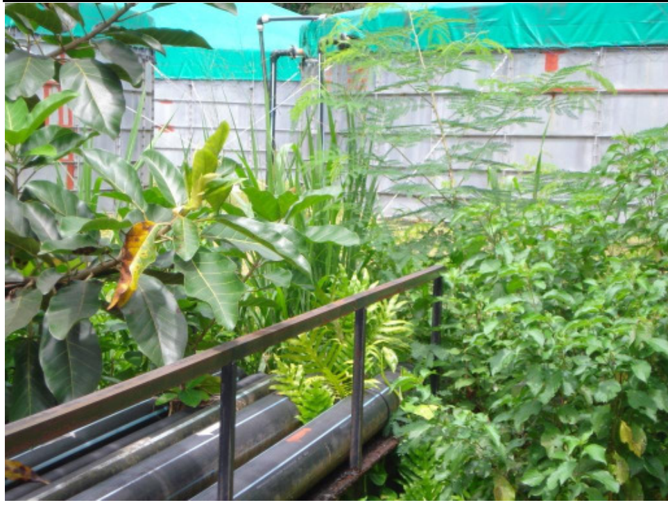
Photo 11 Fresh and grey Water Storage Tanks
