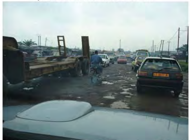
Photo 5.5.12 Significant potholes at Bonaberi Market
