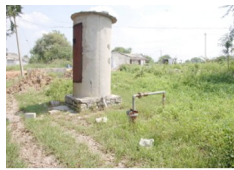
Chatrasala – Water Supply
