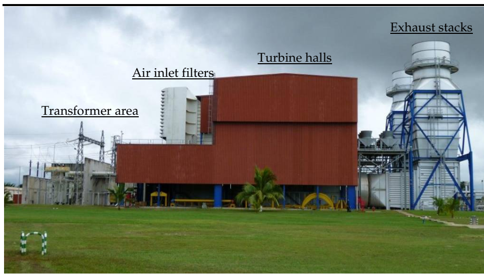
Figure 2.3 Existing Azito facility (turbine halls and exhaust stacks)
