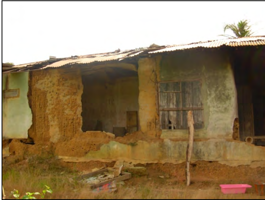
Figure 7-14: One of the houses with broken wall within camp 2.
