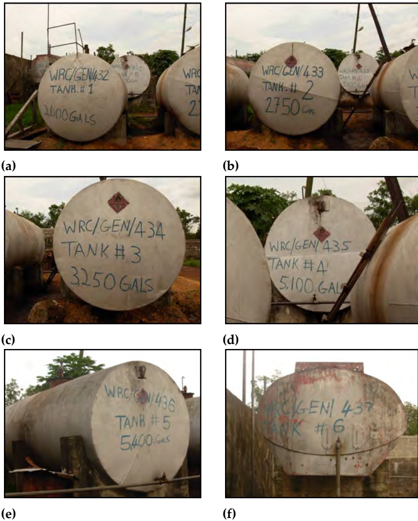
Figure 4-3: Fuel storage tanks. (a) tank # 1 with capacity 2600 gals; (b) tank # with capacity of 2750; (c) tank # 3 with storage capacity of 3250 gals; (d) tank # 4 with storage capacity of 5100 gals; (e) tank # 5 with storage capacity of 5400 gals; (f) tank # 6 currently not used.
