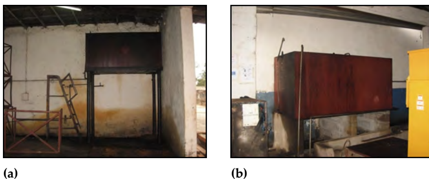
Figure 4-4: Short term storage tanks. (a) Located with the processing plant for the dryer and (b) located within the power plant for the generators.
