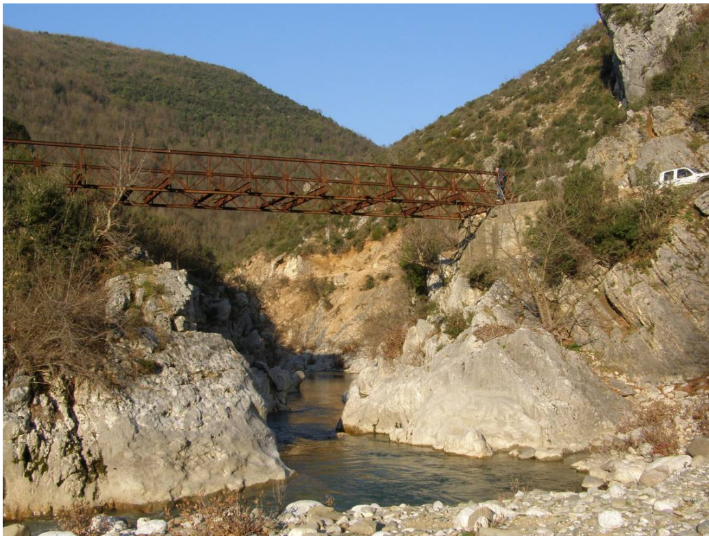
Figure 42 River Drojes Bridge – Deck Destroyed
